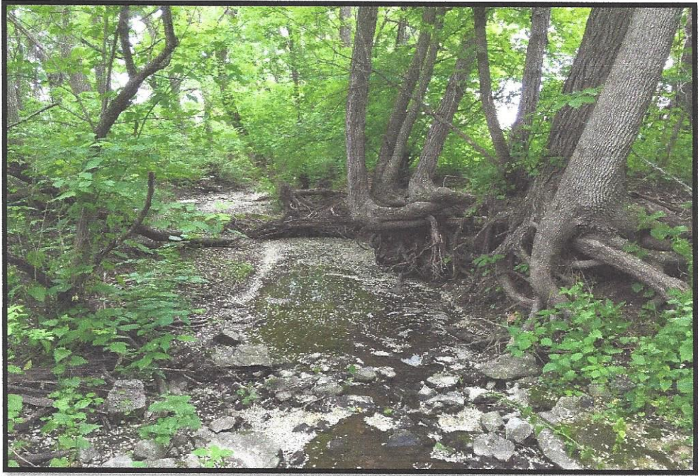
Photo 15 – Bank erosion Reach 2 at upstream end of Brummel Property
