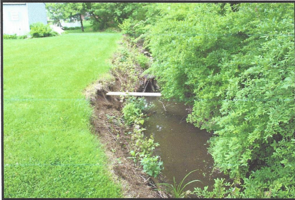
Photo 4 – Bank erosion along upper Reach 2A. Sump pump outfall pipe exposed by erosion. When first installed, only 6 inches of the pipe was exposed.
