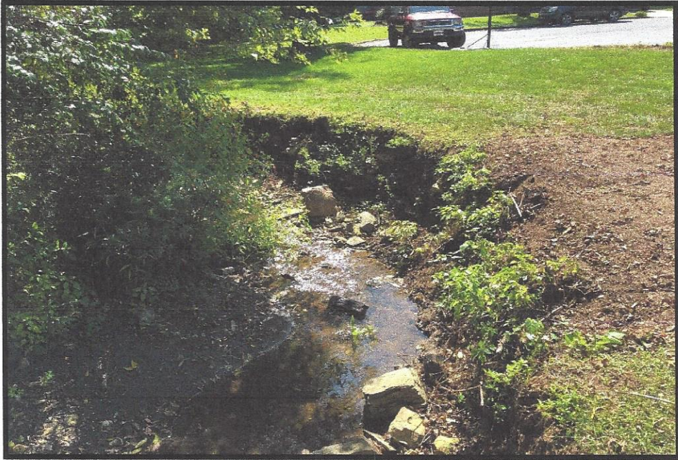
Photo 3 – Bank erosion at Cedar Street Cul-de-sac.
